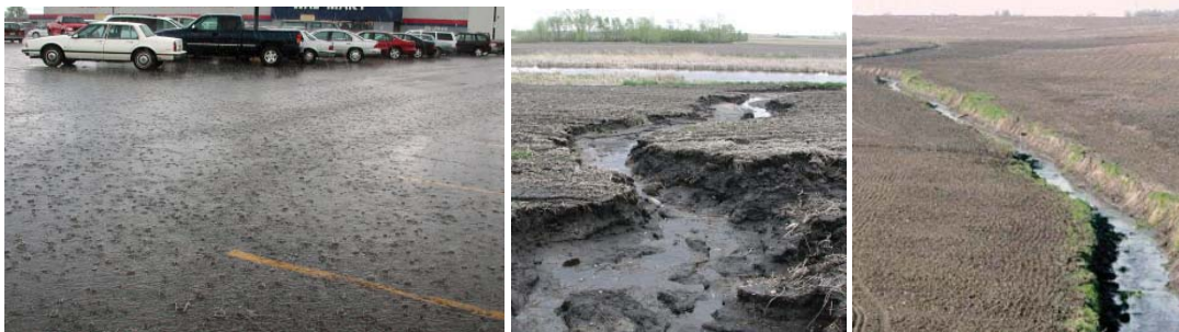
Land use: (above) Parking lot runoff, (bottom center) eroded fields, and (bottom right) unvegetated ditches transport pollutants and excess sediment to streams. Dams and culverts: (top left) A handmade dam disconnects fish from upstream migration and alters the streamflow. (top right) A perched culvert also inhibits fish passage and disrupts the longitudinal connectivity of the stream.
